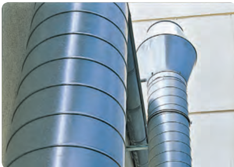
Extract air pipe with deflector hood
