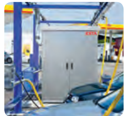
Weather-resistant housing for outdoor installation
