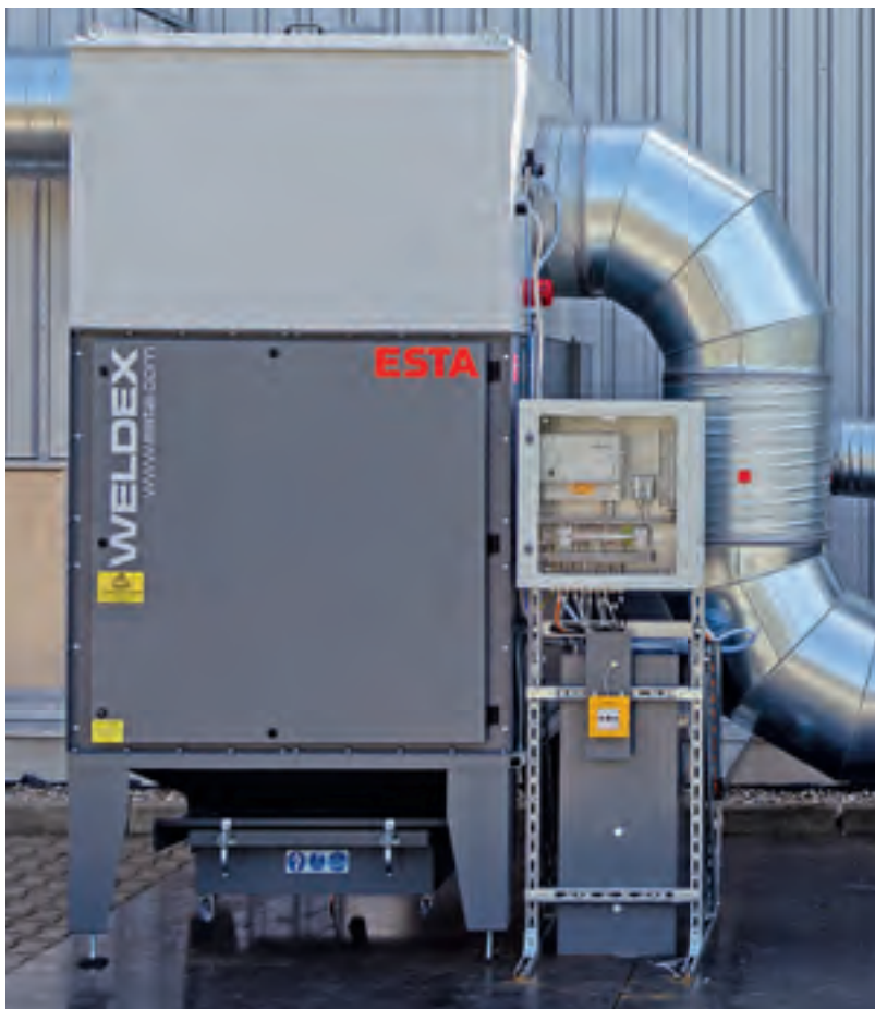
Central filter unit with extinguishing system in a welding fume extraction system
