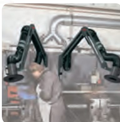
Extraction arm at a welding station
