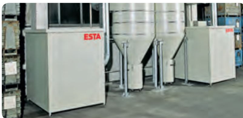
High pressure fans combined with ESTA filter cyclones
