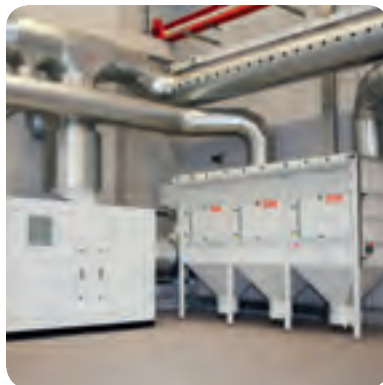
DUSTMAC Filtration unit with Extraction fan and Supply air fan
