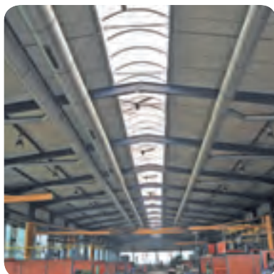
Pipeline system in the production hall
