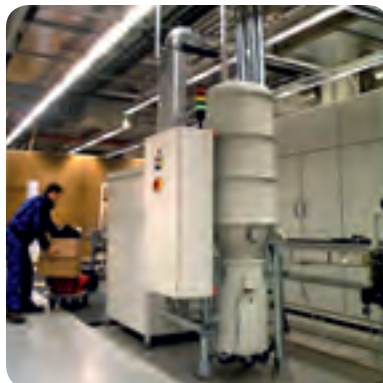
Cyclonic filter FZ-1003 with 100Litre collection container
