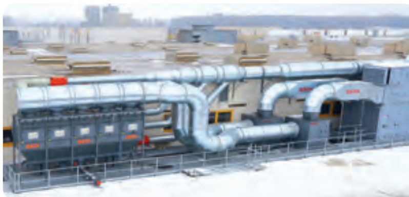
Hall ventilation system on the roof of the production hall
