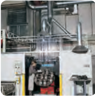
Extraction at a robotic welding station
