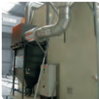
DUSTMAC filter unit on sanding station
