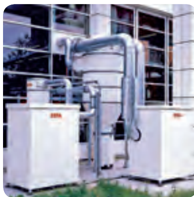
Extraction system with custom paint finish positioned outside
