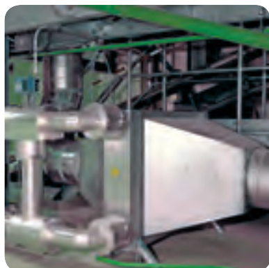
Pipe system for exhaust air with integrated cooling system
