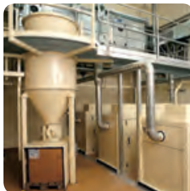
Filter system with dust removal through rotary valves and parallel operating rotary piston blowers
