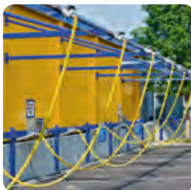
A rigid pipe installation connects the vacuum locations with the cyclonic filter
