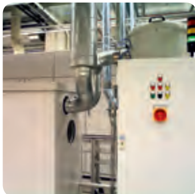
Control unit with monitoring lamps
