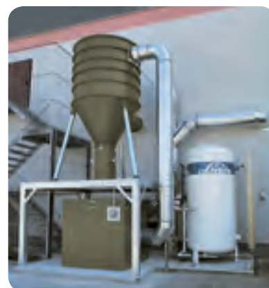
Two cyclonic filters as part of an extraction system
