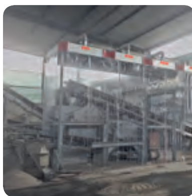
Extraction hoods over conveyor belts
