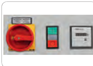
Control panel with operating hour meter
