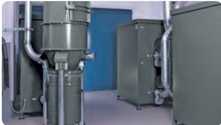
Central vacuum unit equipped with two side channel blowers
